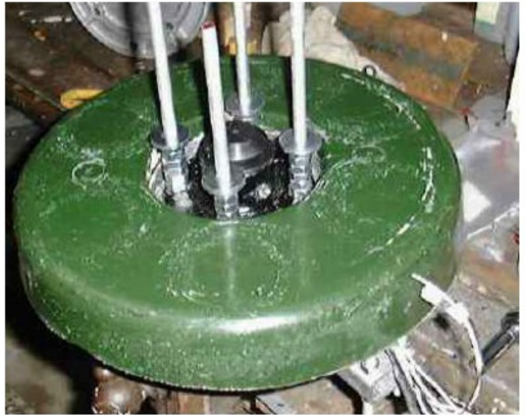
Fitting the stator
